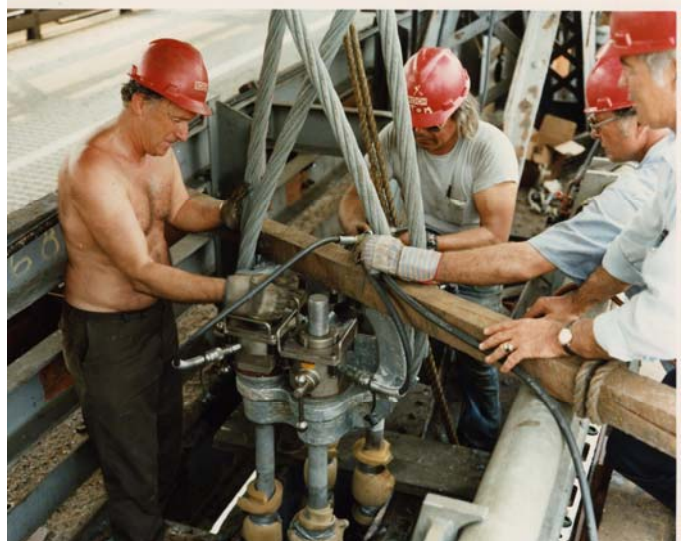
Picture depicts Koch Erecting Co. performing bridge refurbishment on the Williamsburg Bridge using a Biach tensioner.
