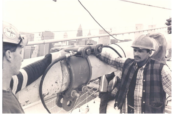
Contractors demonstrate use of bolt tensioning equipment on the Brooklyn Bridge in New York
